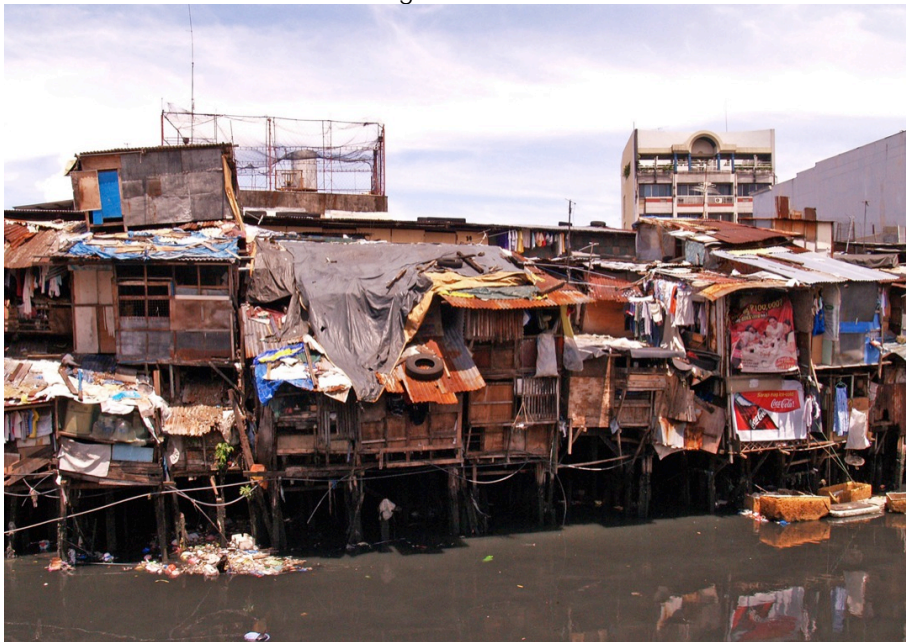
Figure 7 Tondo, Manila, Philippines, 2008 Some informal settlements cannot be upgraded without wholesale demolition.
